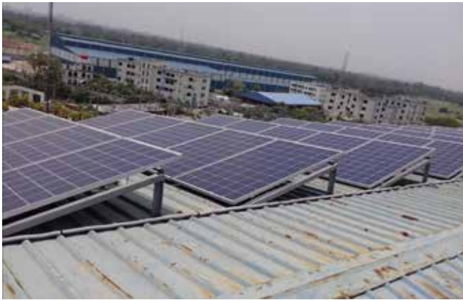
Solar panels at Lolati Factory
